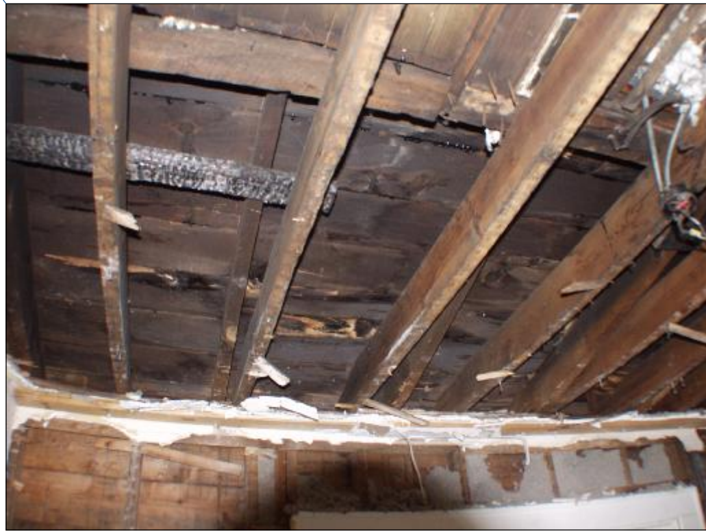
SHOWING OLD SHED ROOF UNDER INCORRECT PITCHED GABLE NOTE-FIRE DAMAGE
