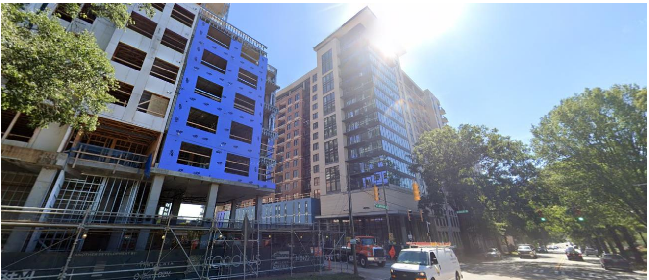
View of high-rise residential buildings under construction located across Morehead Street, northeast of the subject site. The properties are zoned MUDD-O (Mixed-Use Development District, optional) and designated as the Community Activity Center by the 2040 Policy Map.
