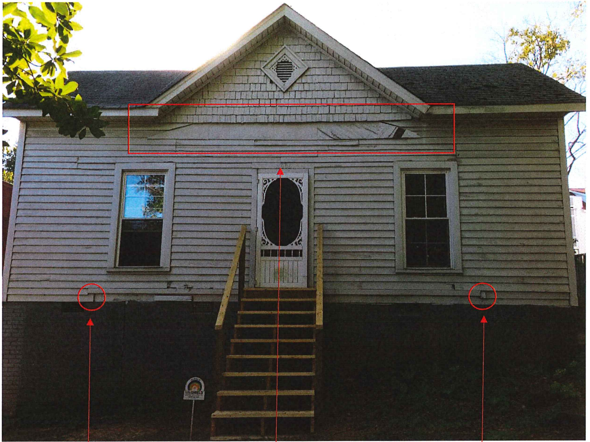
Former porch location, as seen in picture above from inside crawl space
