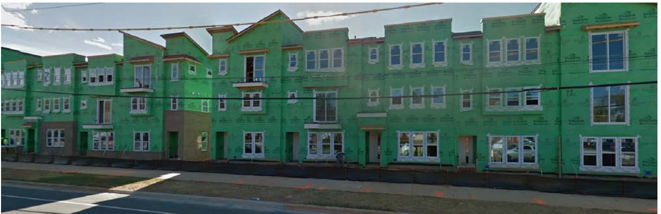
New apartments are under construction along Statesville Avenue to the south of the subject property.
