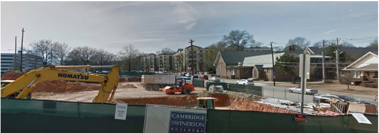
The property to the south is under construction with 380 dwelling units and commercial uses.
