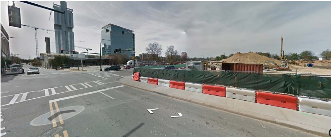
Several sites along Stonewall Street, including the site across South Tryon Street, west of the site are under construction for office, residential and retail developments.
