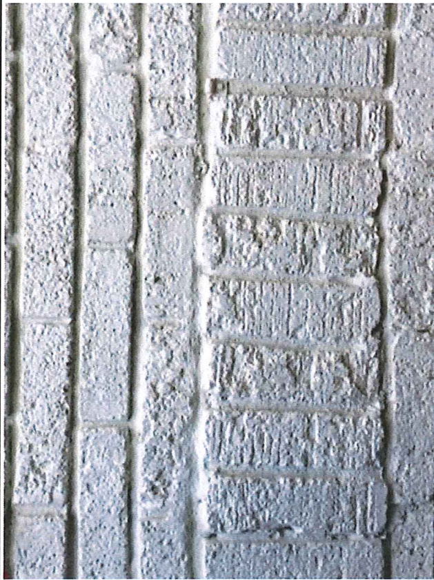
Crooked soldier course. NW wall of 2006 addition. Also note mortar overflow and drips.
